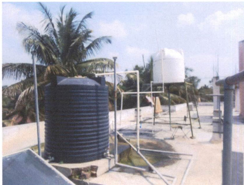
Water storage sump (girls hostel)
