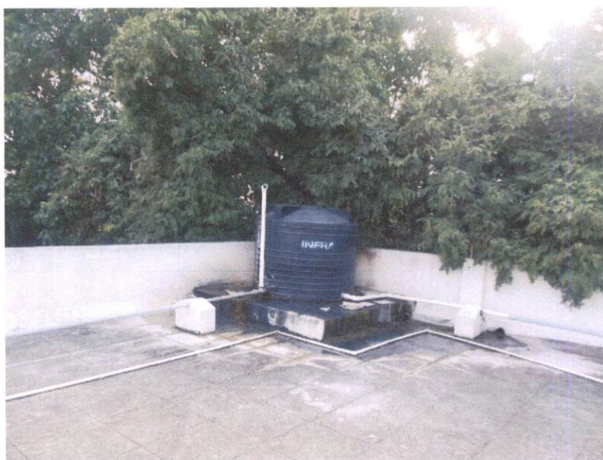
Overhead water storage tank located at boys hostel (block III)
