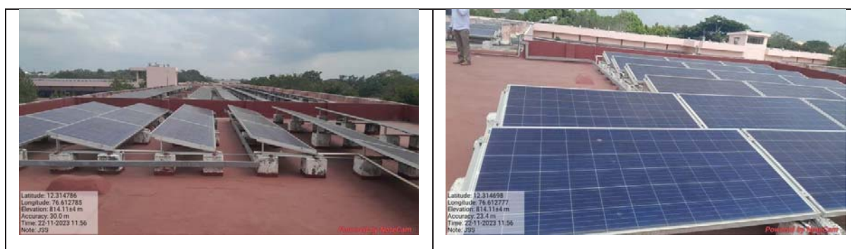
FIGURE 7: PHOTOGRAPHS OF THE SOLAR PANEL
