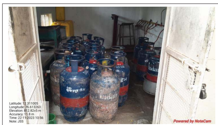
FIGURE 6: PHOTOGRAPHS OF THE LPG ROOM
